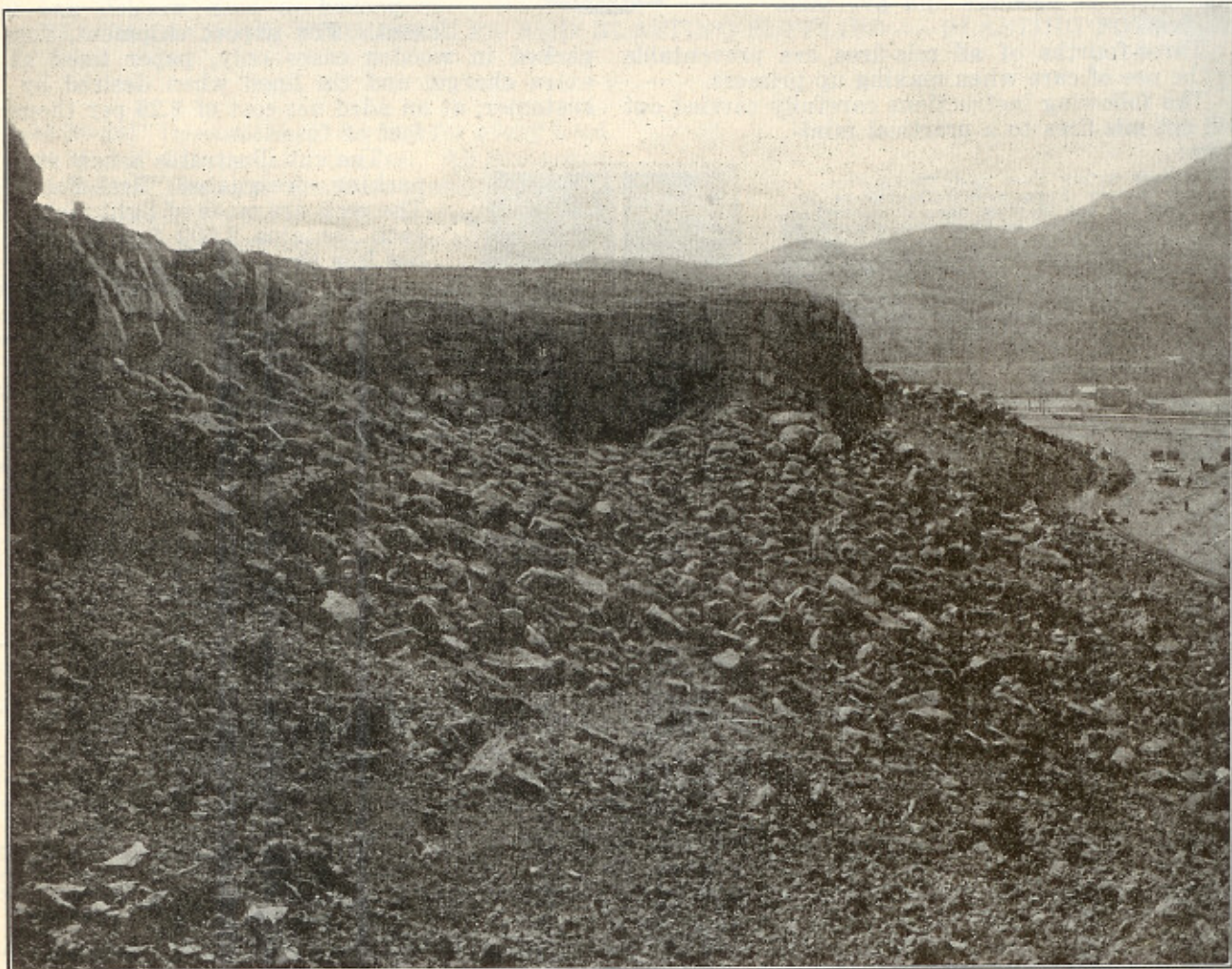
Cordeau-Bickford was used to detonate the 62,350 lbs. of explosive used in this blast. Tonnage of cement rock broken, 370,000.
